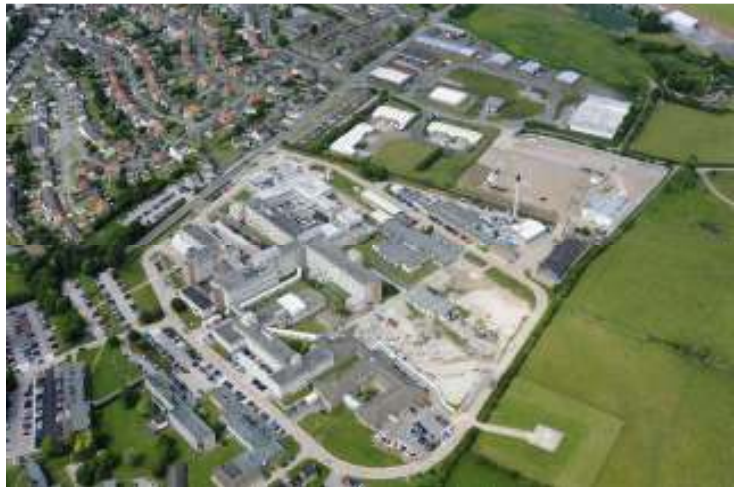
An aerial photo showing the demolition which had taken place at West Cumberland Hospital by July 2010
